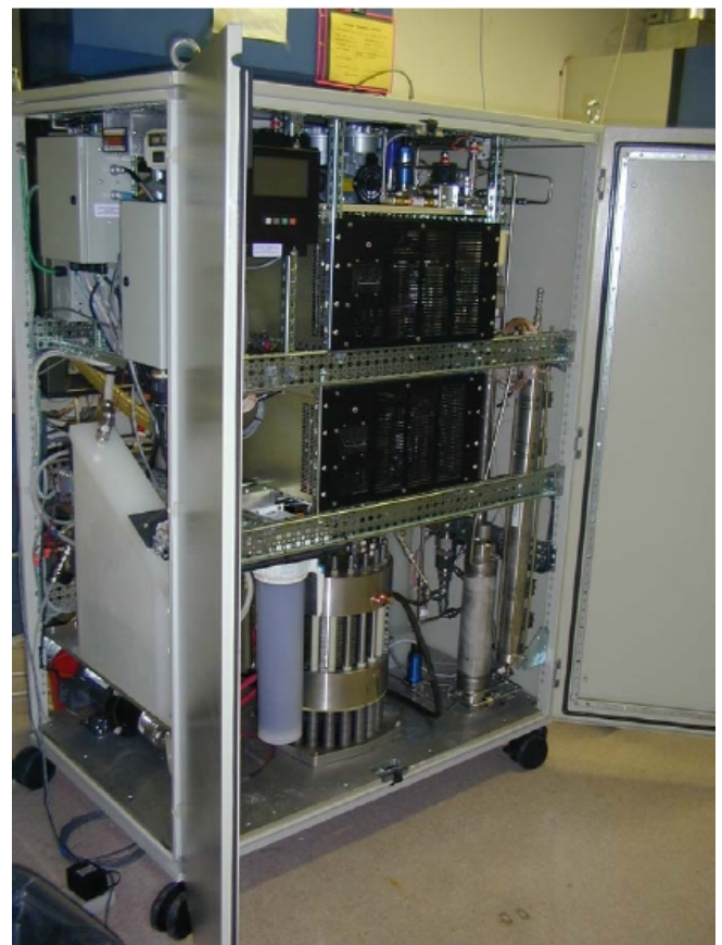
PEM high pressure electrolyzer system
