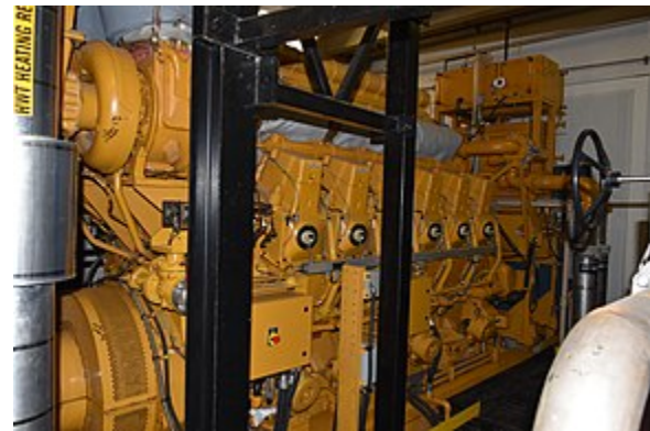
Stationary 12 cylinder turbo-diesel engine coupled to a generator set for auxiliary power
