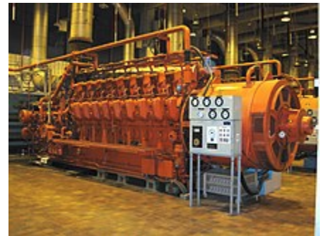
Diesel generator for backup power
