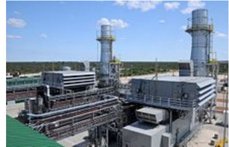
Turbine power plant
