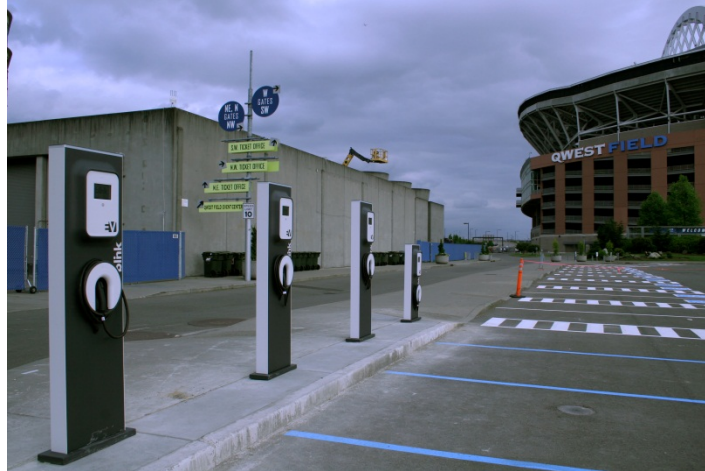
Figure 10. Typical alternating current Level 2 public charging station.
