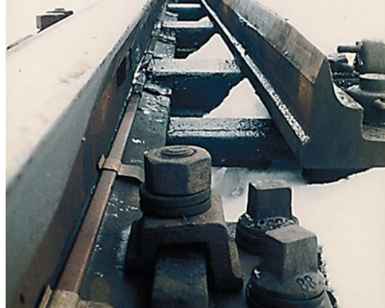
Figure 2: Railway switch equipped with electrical heater. Source: railway-technology.com.
