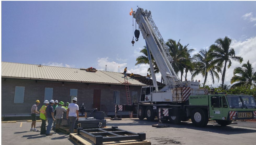
Makai installed advanced manufacturing equipment to be used to produce marine-grade heat exchangers at our Ocean Energy Research Center. Installation required removing part of the roof!
