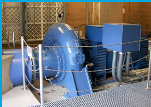
Ponderosa Hydropower Project Photo courtesy Gary Johnson, Pacific Northwest National Laboratory
