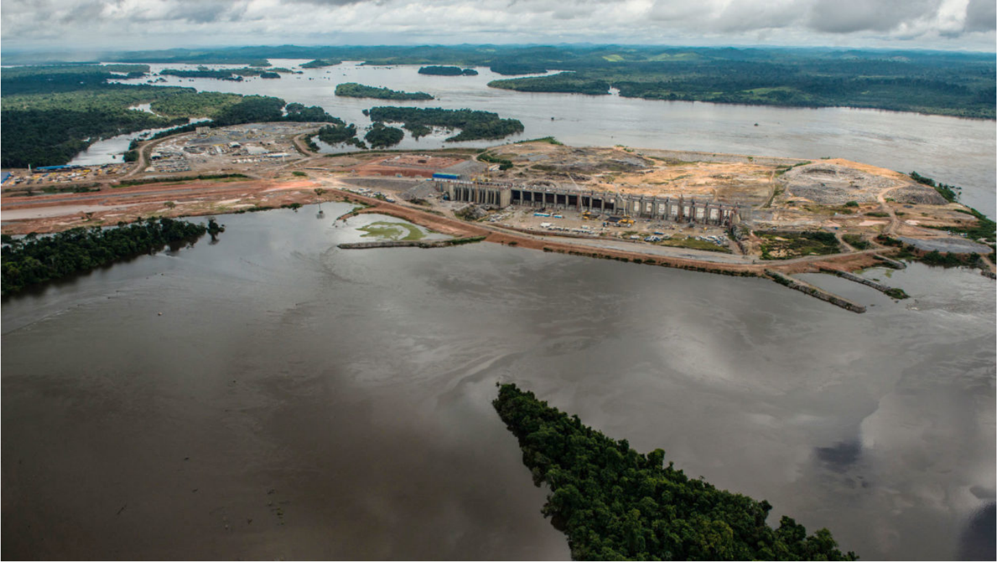
The Belo Monte Dam under construction on the Xingu River, a tributary of the Amazon, in 2015. FÁBIO NASCIMENTO/GREENPEACE
