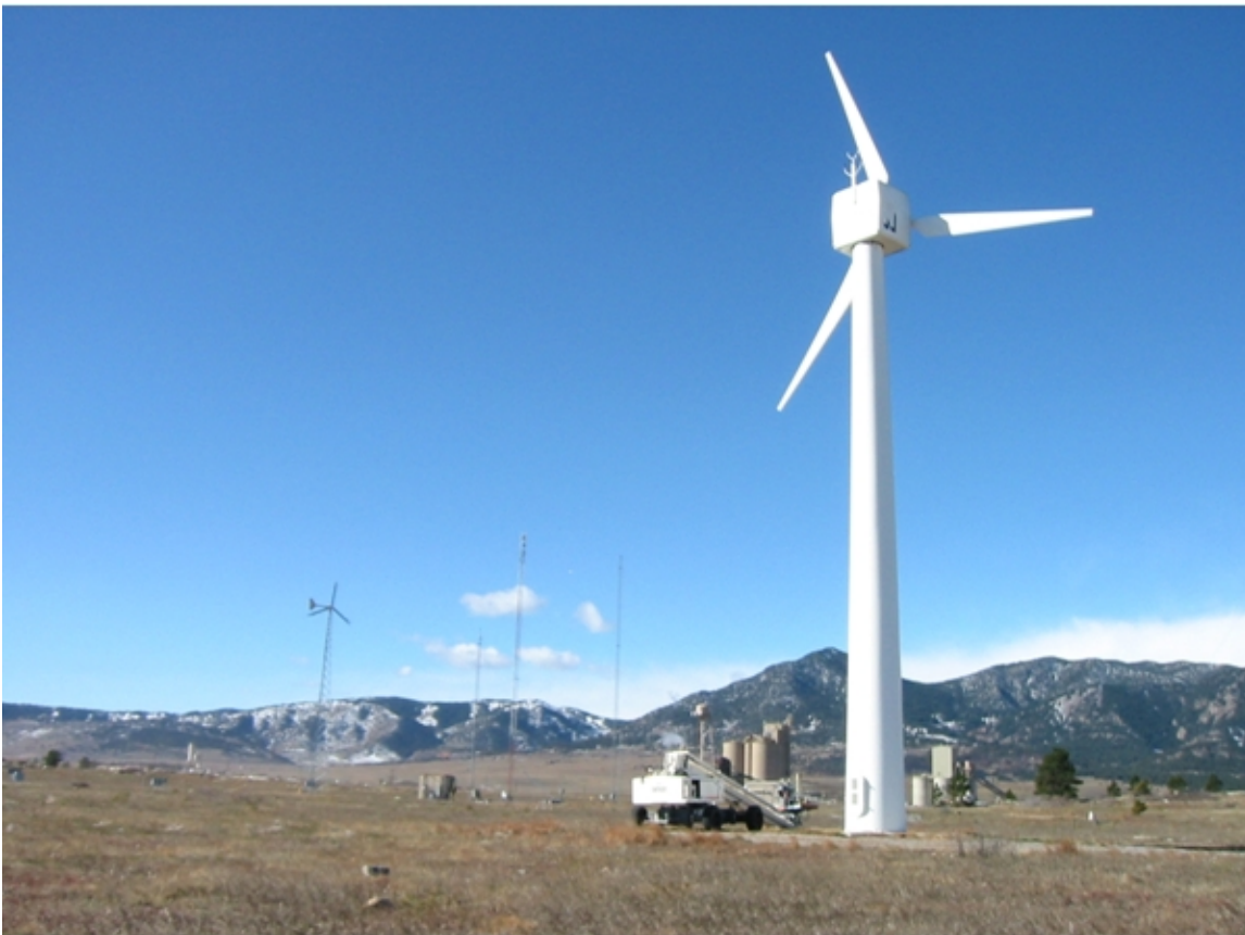
Figure 11. 100-kW wind turbine (NREL 2008)
