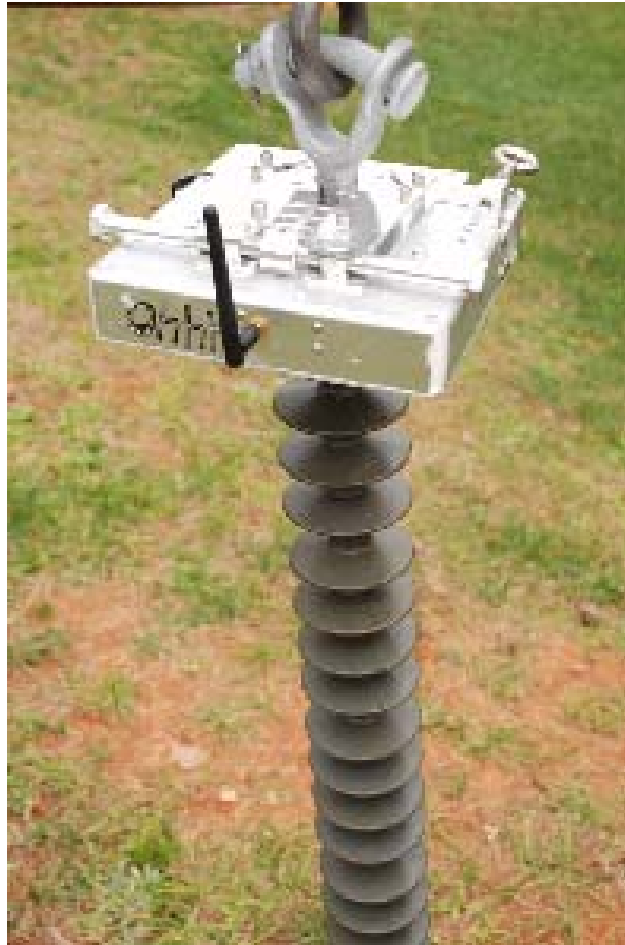
Figure 5-5 Clamp-on RF leakage current sensor for transmission line applications installed on a 115-kV composite insulator.
