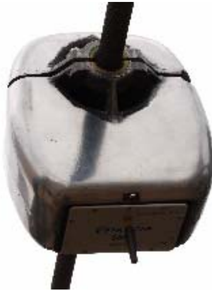
Figure 5-10 Conductor temperature sensors installed on a steel-reinforced aluminum cable (ACSR) conductor. The sensor communicates using a cell phone modem.
