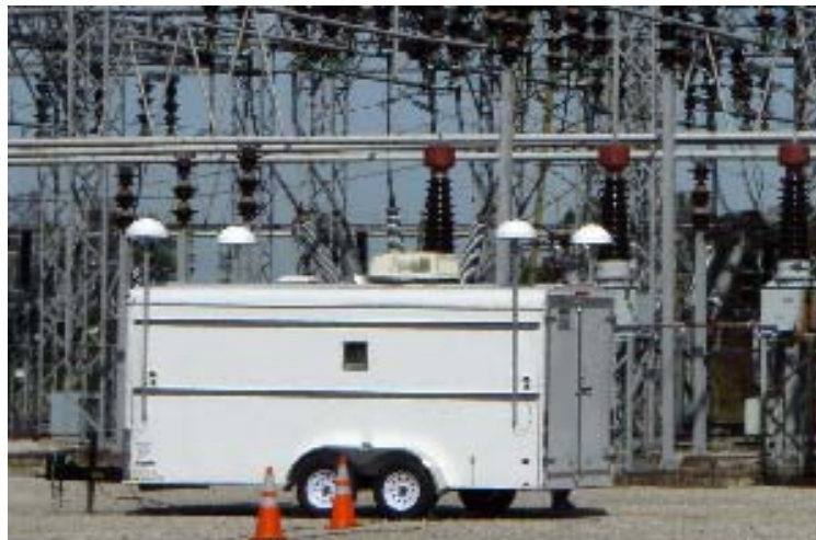
Figure 5-7 Antenna array installed on a portable trailer deployed in a 161-kV substation.
