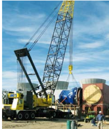
Installing the SST-700 low pressure steam turbine on the Boulder City site, Nevada, USA
