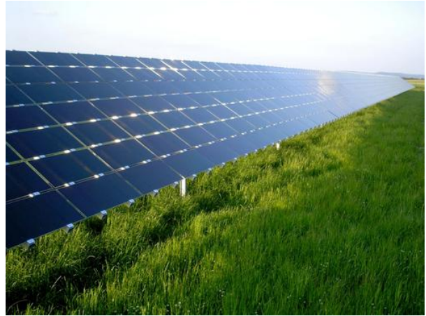
PV array made of cadmium telluride (CdTe) solar panels
