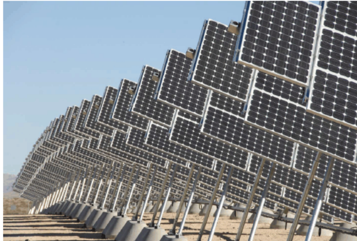
Figure 30. Nellis AFB Photovoltaic Array Detail
